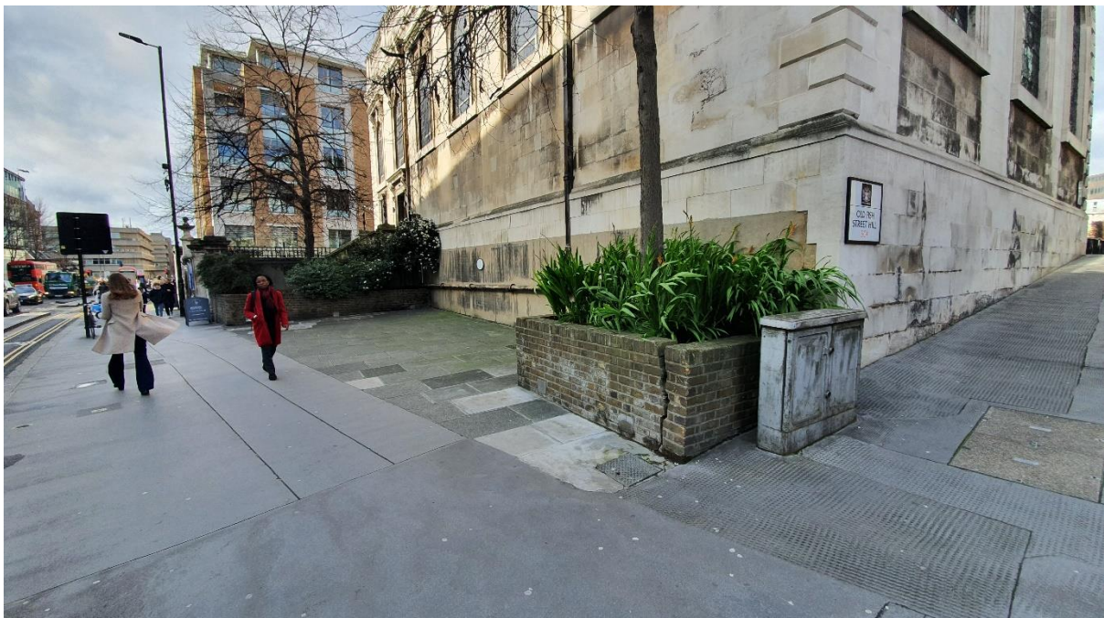
Phase 3 | Damaged planters adjacent to Church to be rebuilt in January 2024 - Existing
